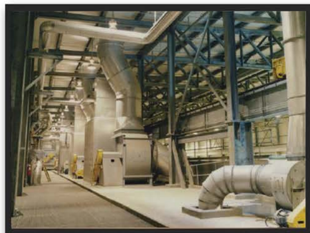
HOOD EXHAUST SYSTEM
